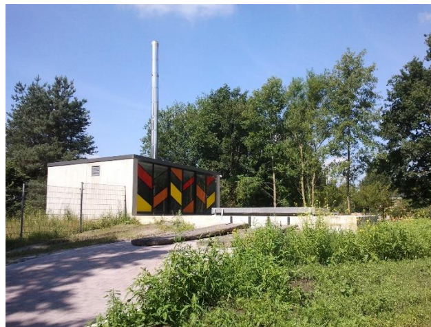
Wood chip fired boiler 500 kW
