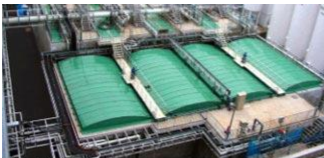
Water Purifying System
